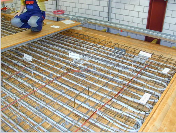
TABS register with steel reinforcement
